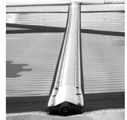
▲ needs batten tension
